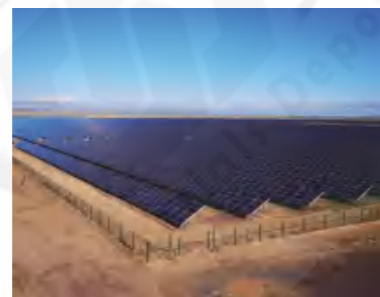
Agadyr Power Plant Kazakhstan System Capacity: 50 MW
