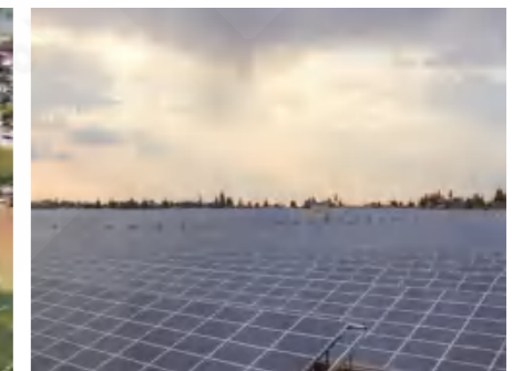
Pavagada Power Plant India System Capacity: 350 MW (Suntech Supplied 210 MW)
