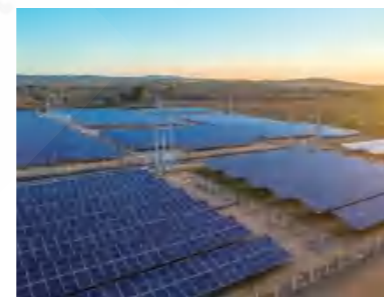
Setta PV Power Station Brazil System Capacity: 1.5 MW
