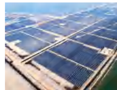
Dongying Double Glass Power Plant China System Capacity: 92 MW
